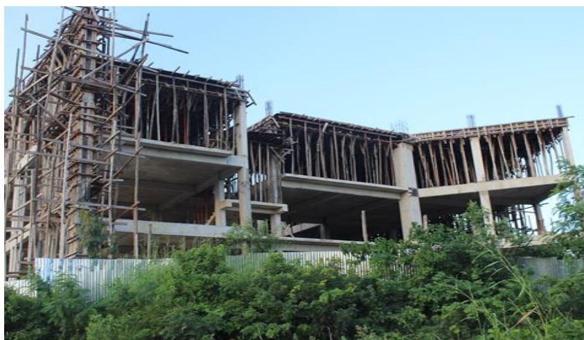
A latest picture of the on-going construction of the Students Centre at the University Main [Mwl. Julius Nyerere] Campus
